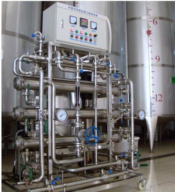
FIGURE 4.2 Picture of the nanofiltration equipment for pilot test.
